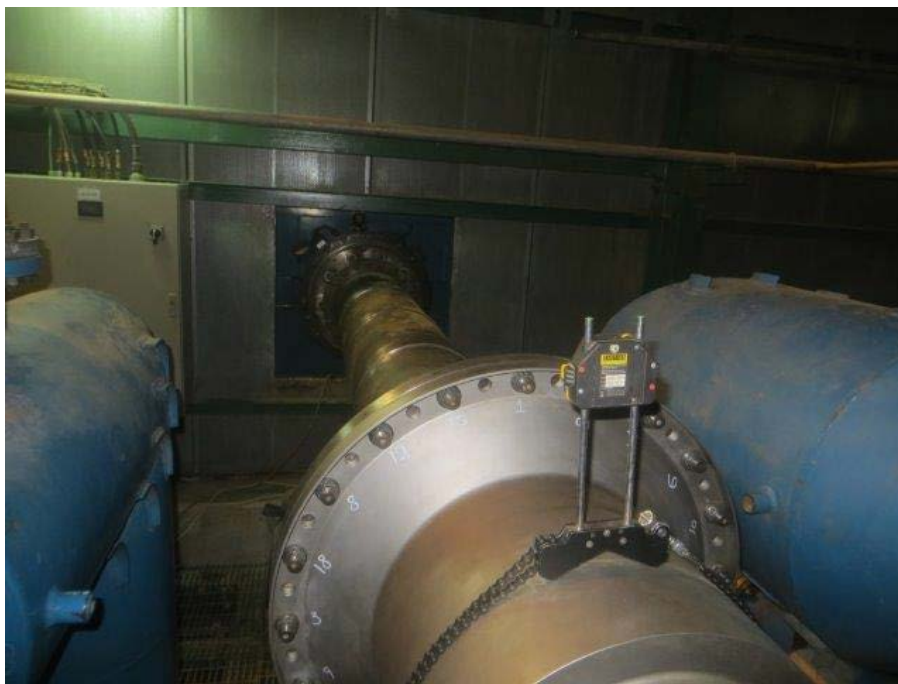
Figure 3. Setup of the laser equipment on one coupling of the spacer shaft facing the motor.
