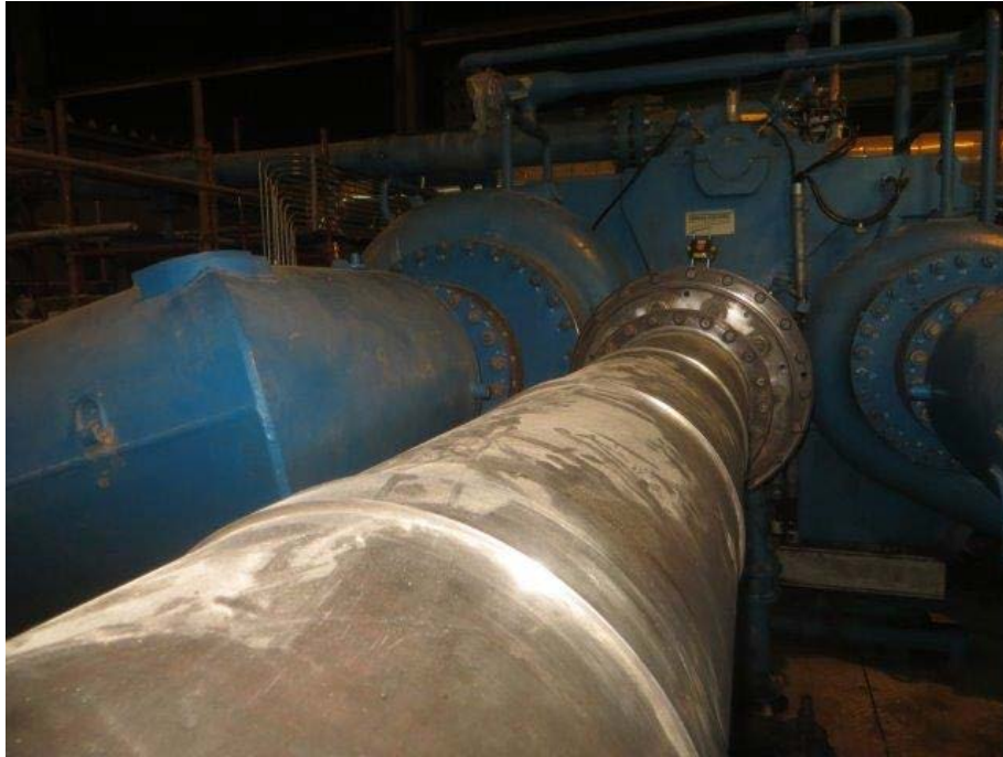
Figure 4. Setup of the laser equipment view from the motor end looking towards the compressor.
