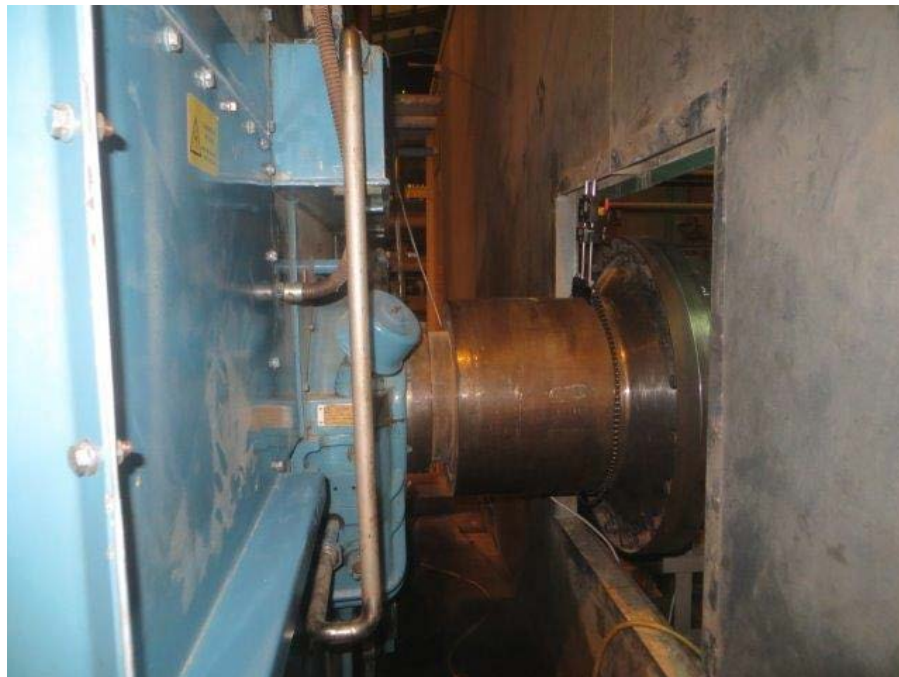
Figure 1. Electric motor on the left with spacer shaft connection thru the sound dampening enclosure.
