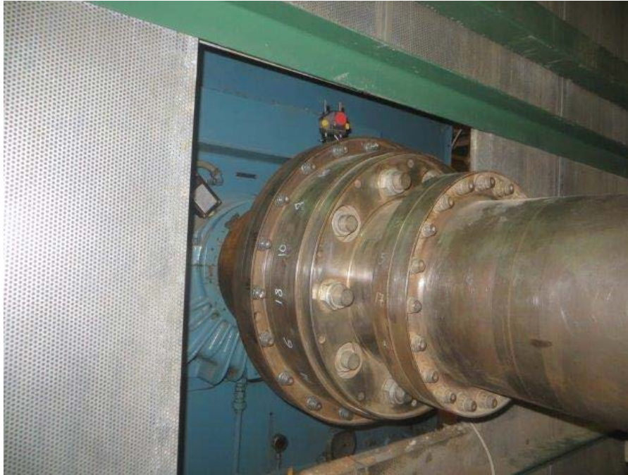
Figure 2. One end of the spacer shaft coupling attached to the motor.
